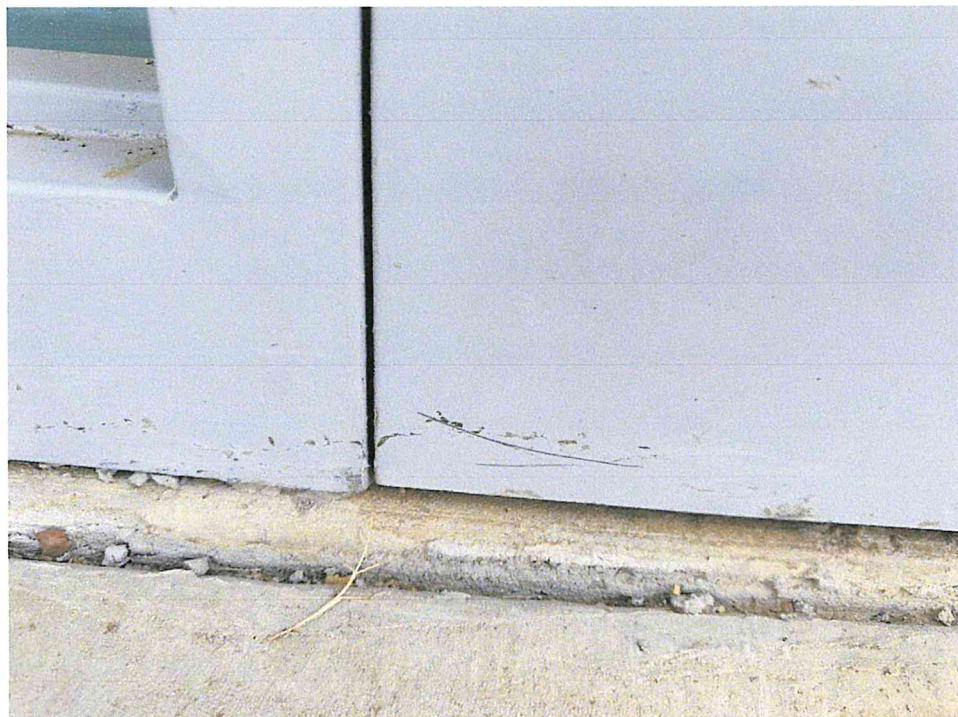
Figure 6 – Repair damaged paint.
