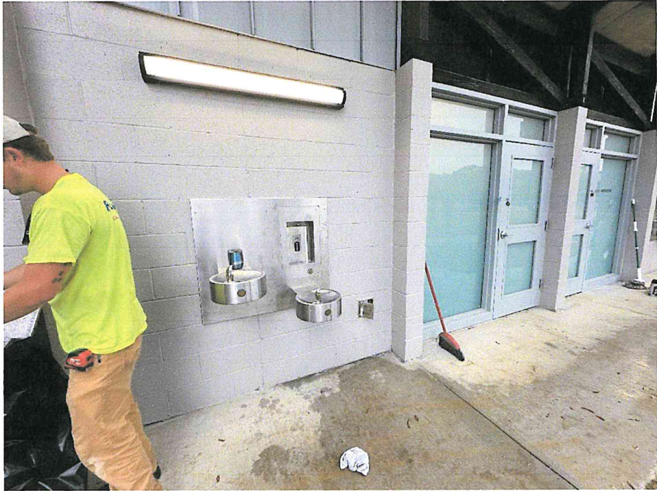
Figure 5 – Water fountain pressure is a little high.
