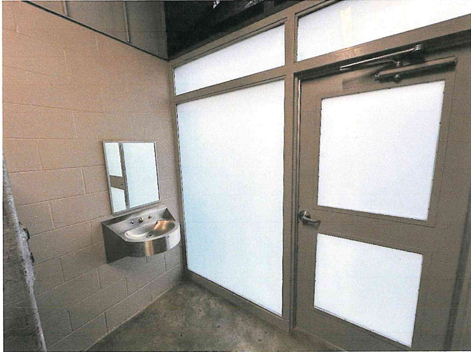
Figure 3 – Closers missing covers throughout
